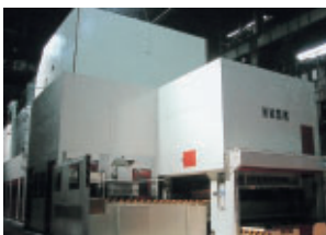
Stamping press equipped with sound insulation (the Second Stamping Section, Yajima Plant, Gunma Manufacturing Div.)
