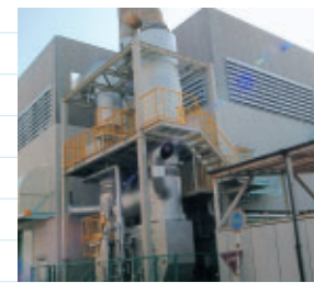
The natural gas cogeneration system introduced at the Utsunomiya Manufacturing Division
