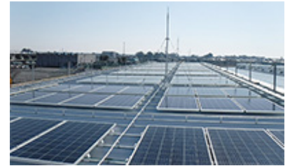
Oizumi Plant of Fuji Machinery Co., Ltd.
