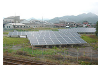
Solar power generation system with the output corresponding to the use by 100 detached houses.
