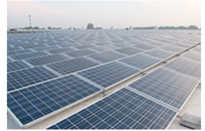
1 MW Power Generation Facility
