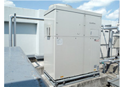
Cogeneration system installed in the Subaru Training Facility
