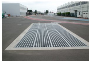
Flood prevention measure (drainage grid) (Utsunomiya Plant)
