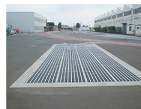
Flood prevention measure (drainage grid) (Utsunomiya Plant)
