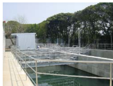
The Main Plant The oil-separating tank of the drainage ditch No.2
