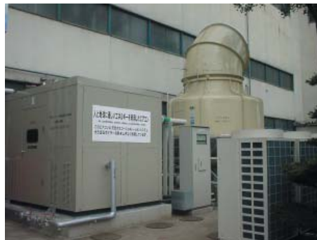
A steam absorption type water cooler and heater: It takes advantage of waste heat to air-condition a part of the plant.
