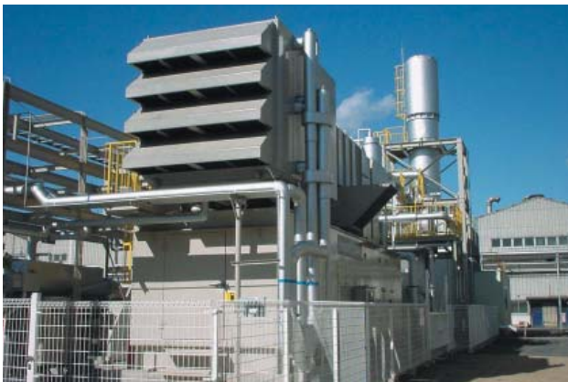
The Cogeneration System in the Yajima Plant
